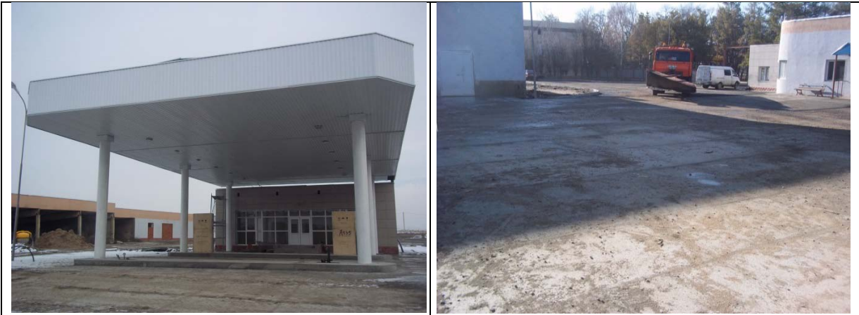
Maintenance depot-34, Petrol station – Process equipment (petrol pumps) (left) and – Land Improvement - Cement concrete pavement (right)
